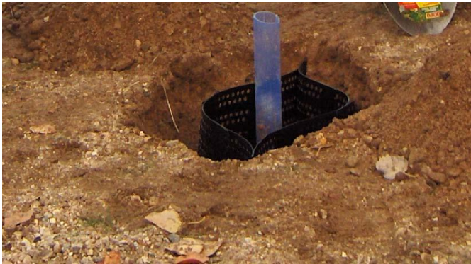
Figure 4: Rigid plastic webbing surrounding a neutron access tube. Completion of tube included the cutting of PVC below land surface, installation of well cap, and backfilling the hole.
